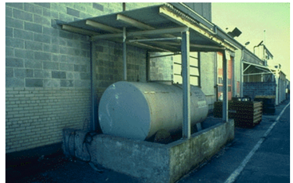
Covered AST with secondary containment
